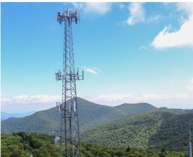
Mt. Pisgah communications tower for electric and internet utilities Photo Credit: Exploring Chatt
